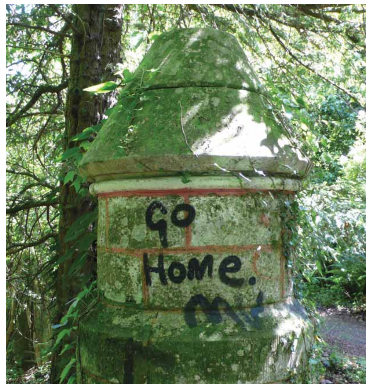
Graffiti Kilmahew main bridge parapet, photograph - Johnny Bute
